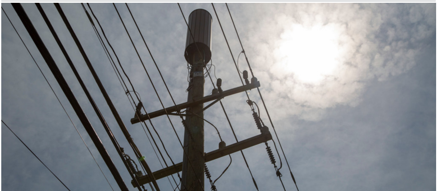
Figure 27. Fibre and 5G assets sharing electric network poles
